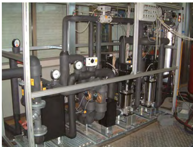
Figure 5. Semi-industrial setup for systematic functional testing of elements needed in the heating and climatisation of buildings. The control system for the setup shown here was developed by the Department of Systems and Control.
